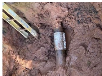
water main break
