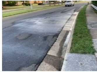
Water Main Break
