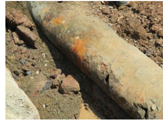
water main break
