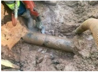
Water Main Break
