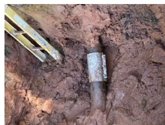
water main break
