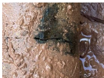
water main break
