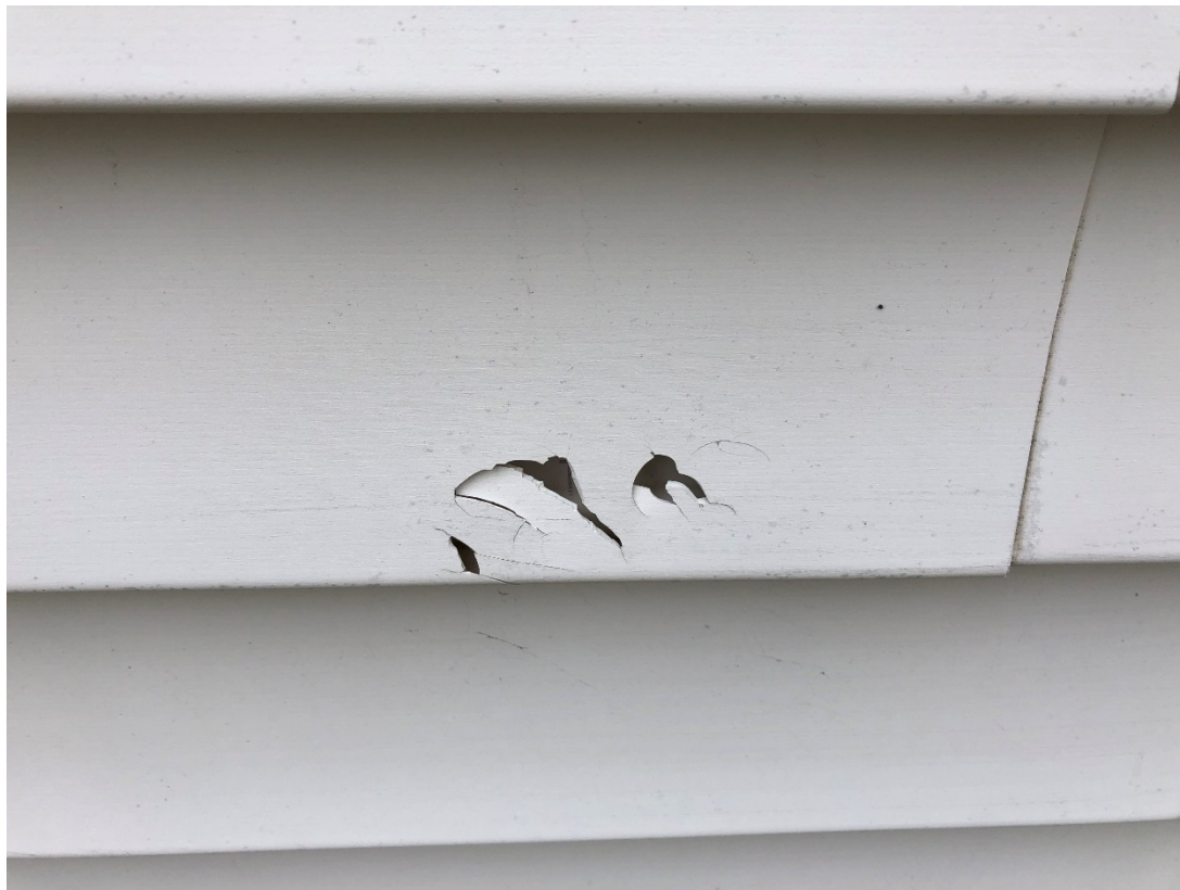
Current brittle damaged siding
