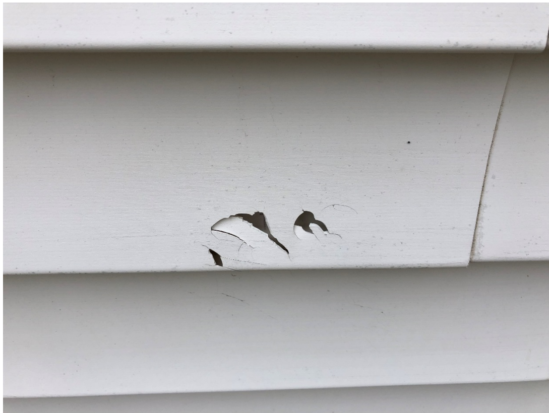
Current brittle damaged siding
