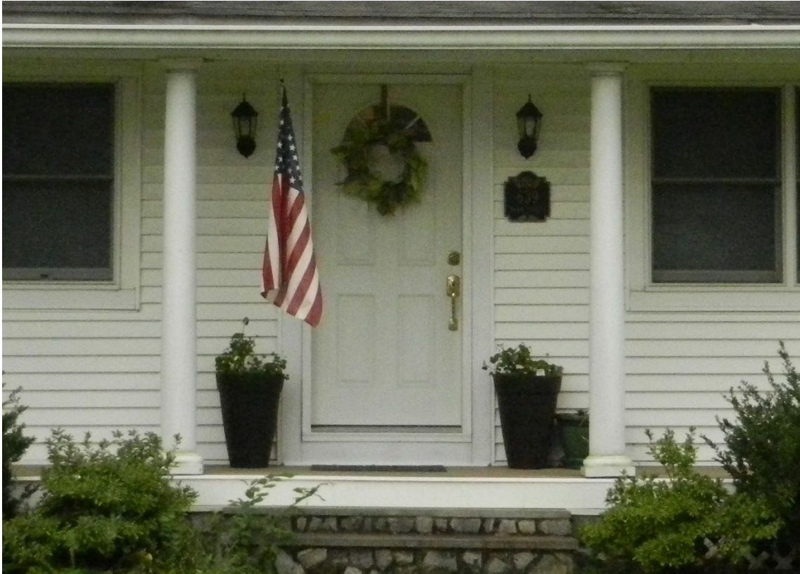
Current tapered columns
