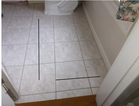
Lines Depict locations of cracks
