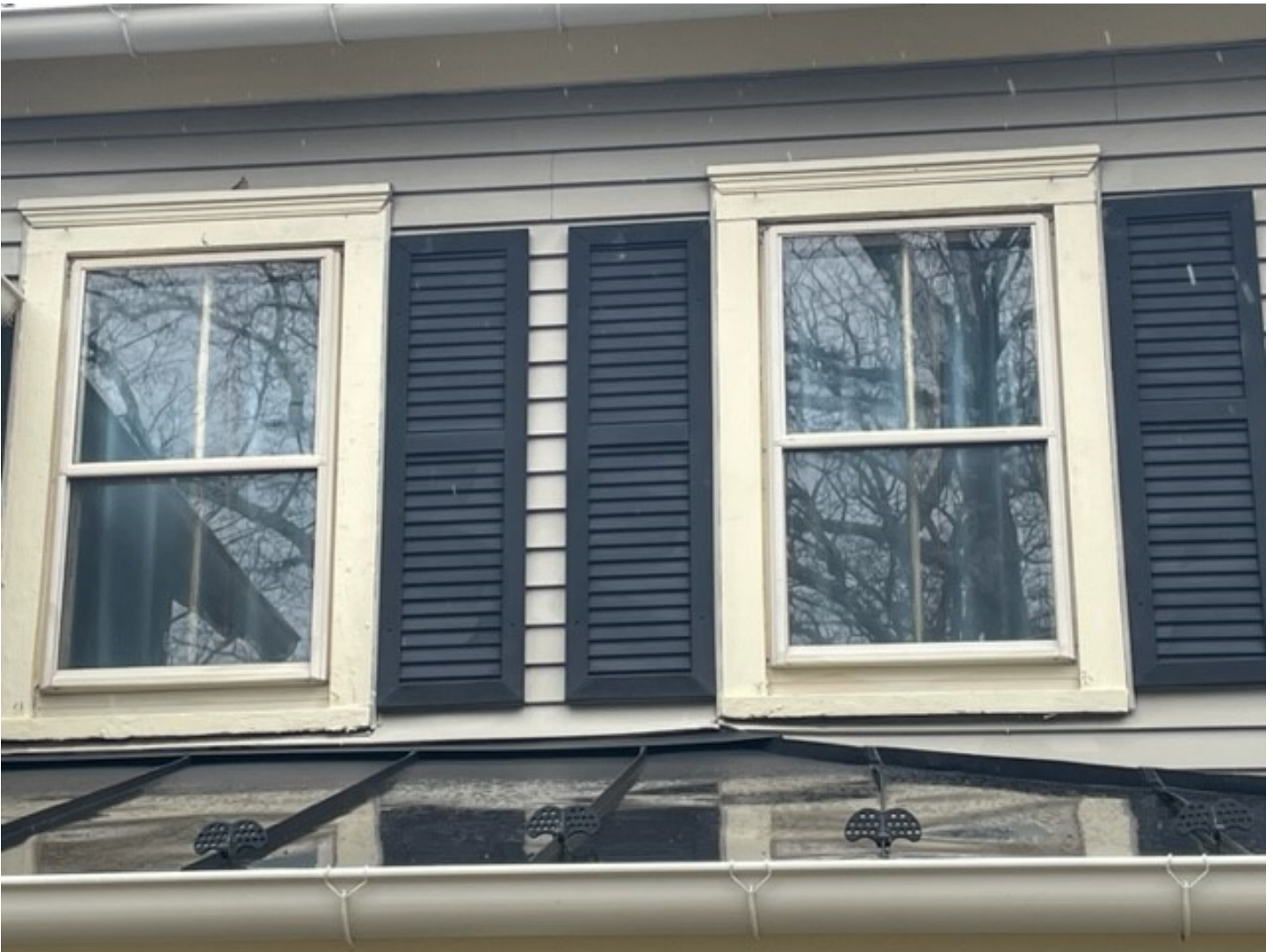
Original windows in home. The goal is to match this design for the new windows.
