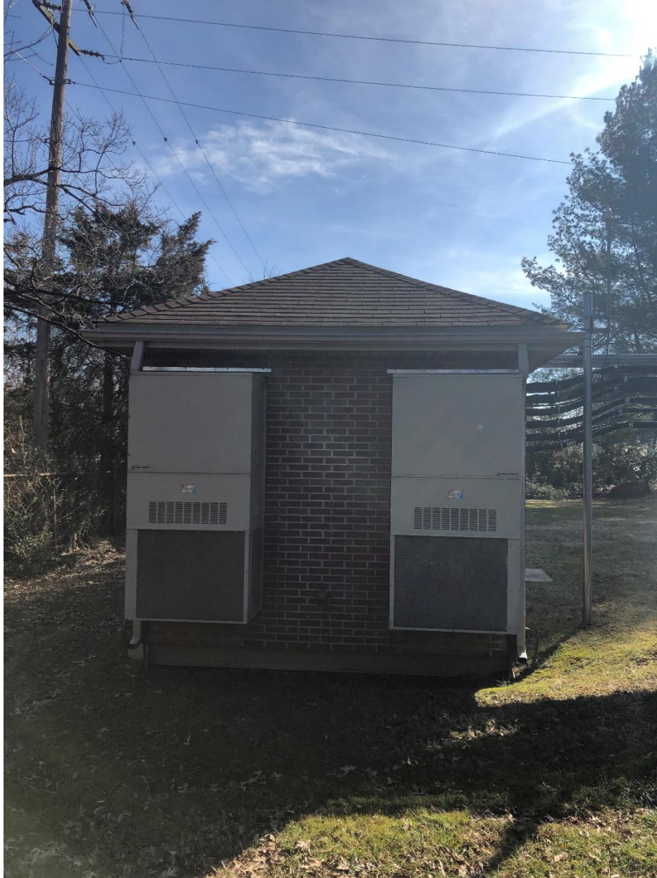
Verizon Equipment Shelter
