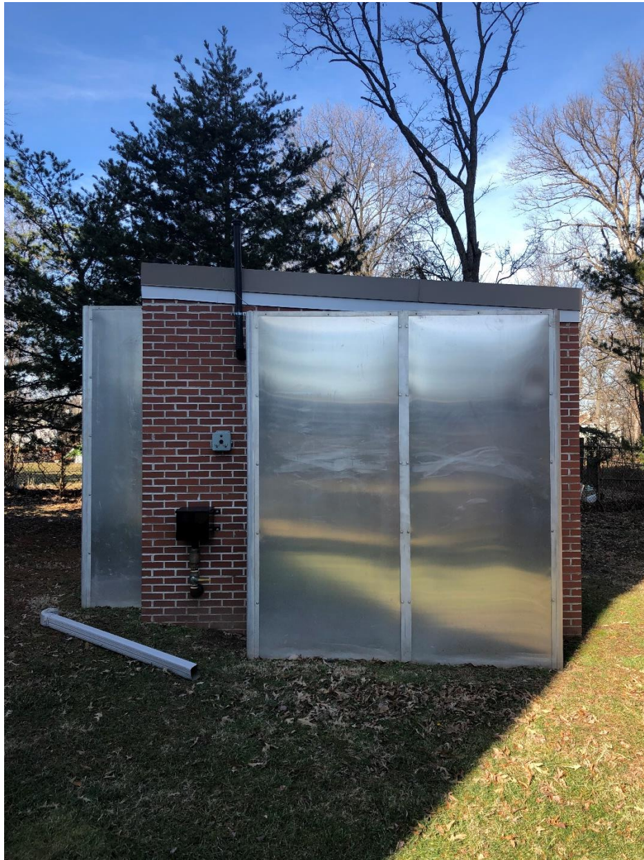
Verizon Generator Stealth Enclosure
