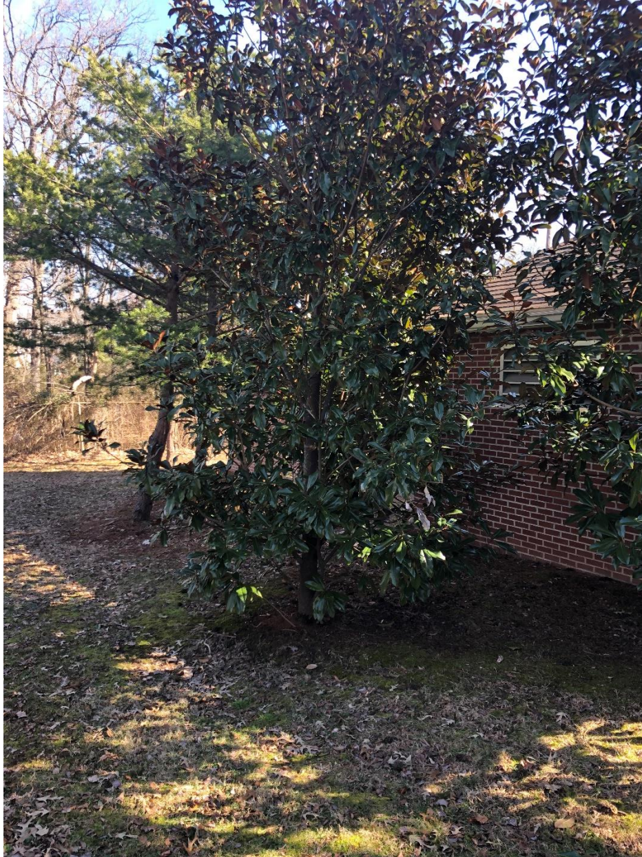
AT&T Equipment Shelter
