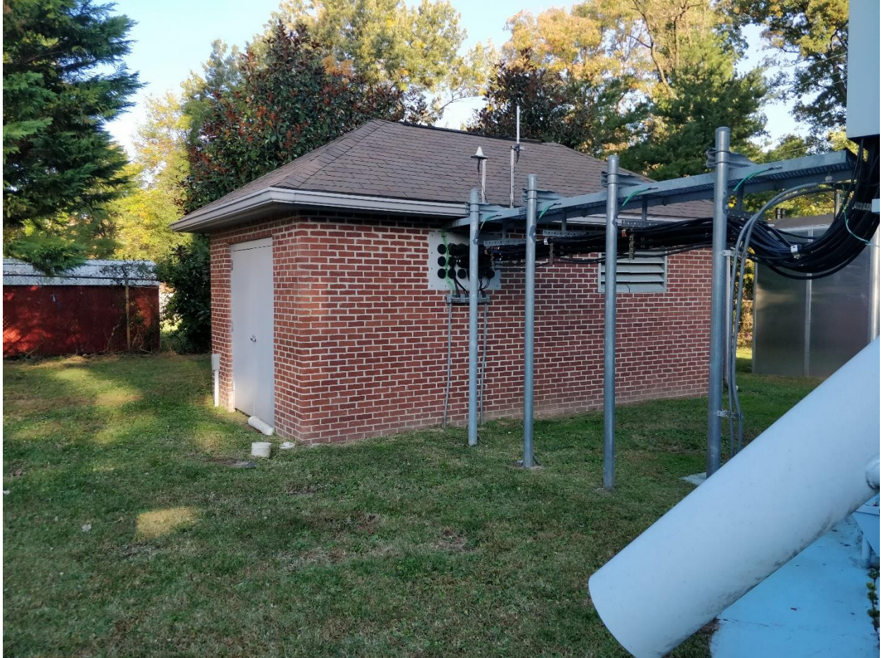
T-Mobile Equipment Shelter
