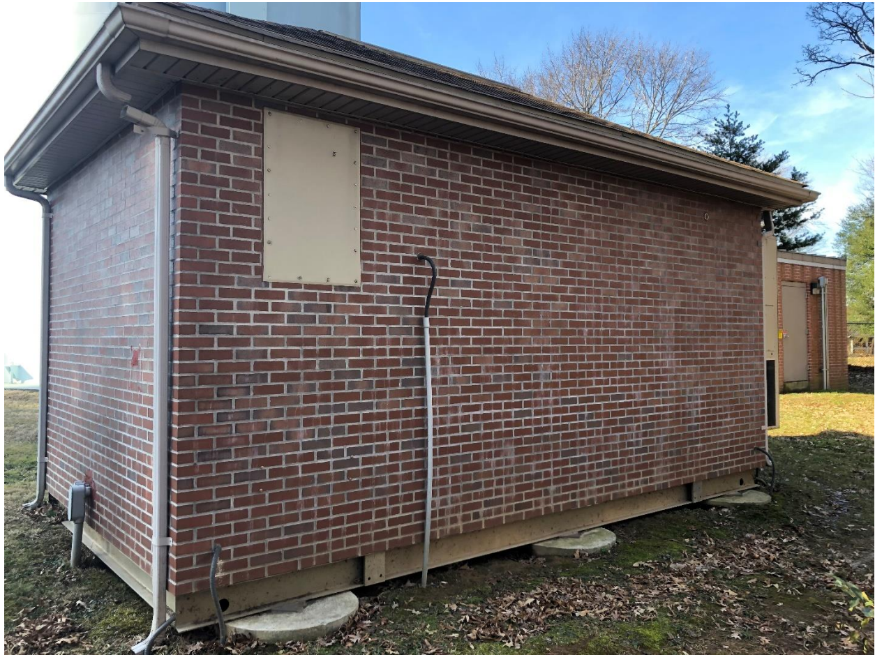
Verizon Equipment Shelter
