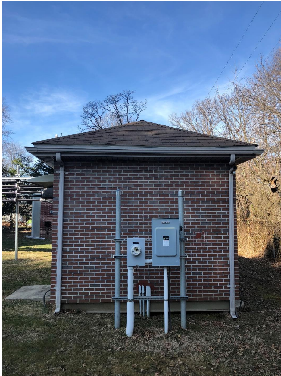
Verizon Equipment Shelter
