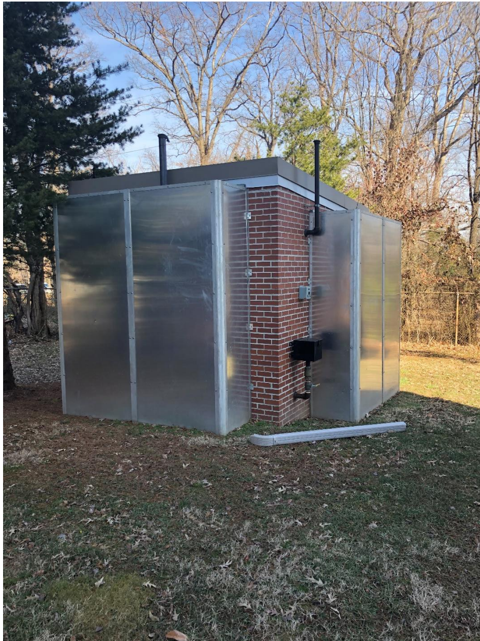
Verizon Generator Stealth Enclosure
