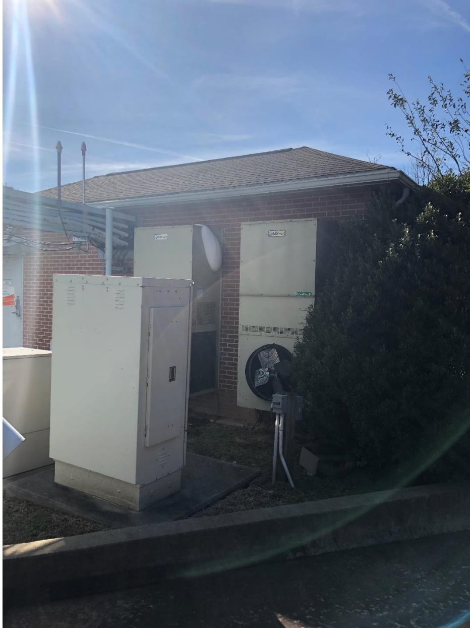
AT&T Equipment Shelter
