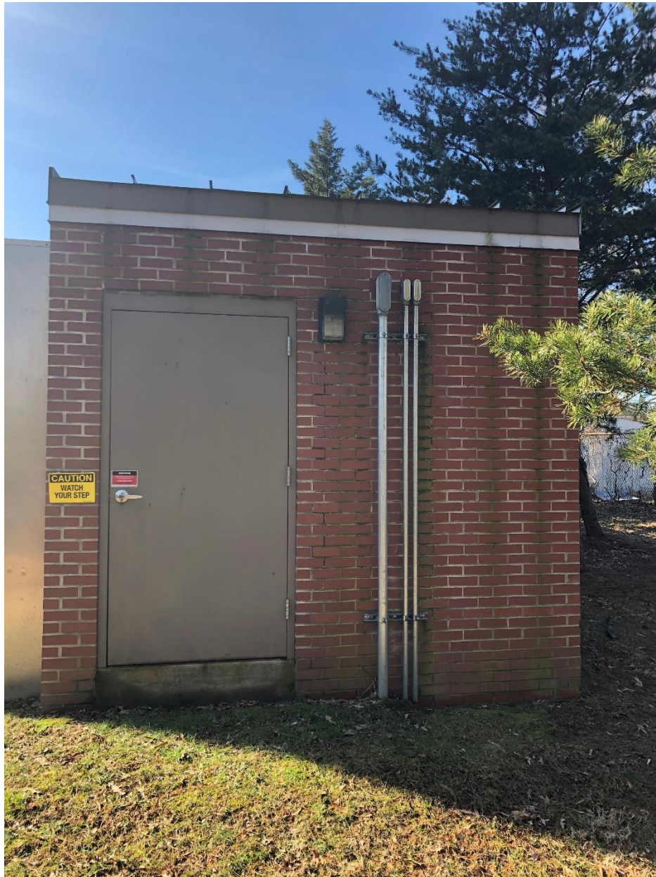
Verizon Generator Stealth Enclosure
