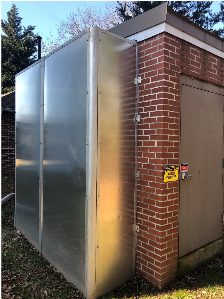
Verizon Generator Stealth Enclosure
