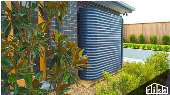
Rainwater harvesting cistern
