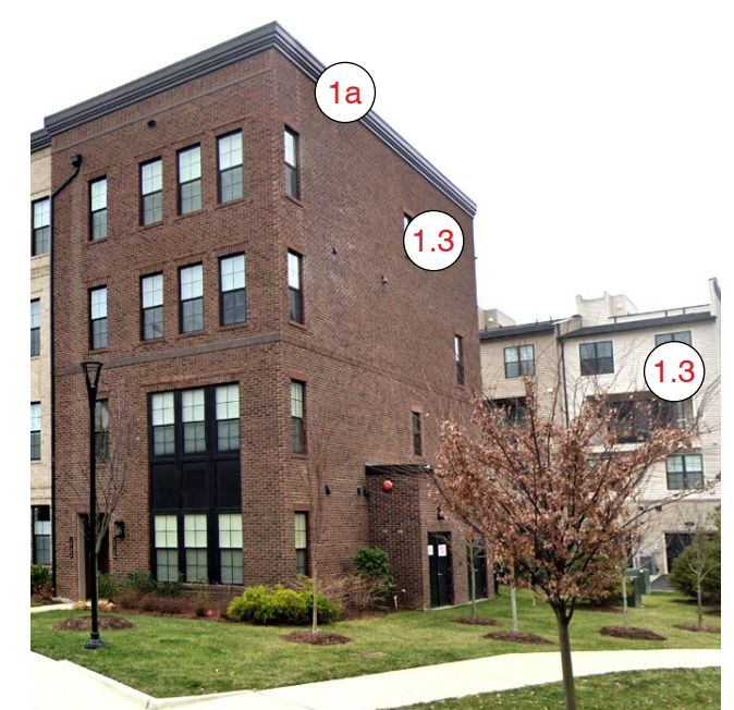
1.a FLAT ROOF with PARAPET Shed style roof is concealed by the parapet at front & side (shed at back is exposed)
