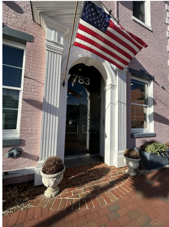
Figure 3: Detail of the existing glass double doors and transom at 783 Station Street.
